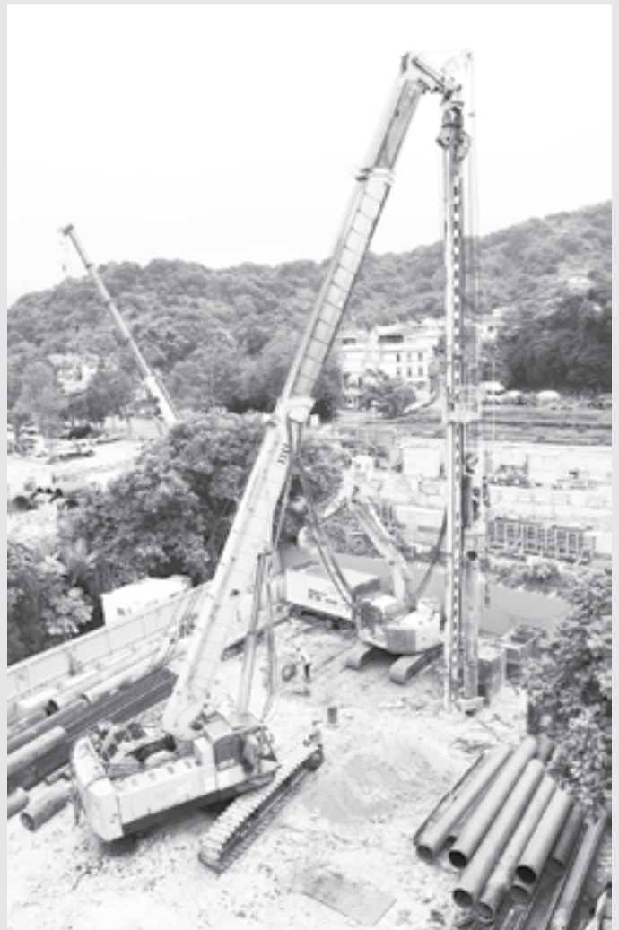
Preparation work for piling is being done at the new building’s construction site.
